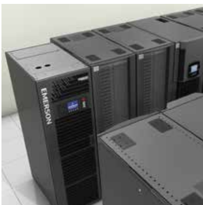
Liebert eXM detached from the wall
